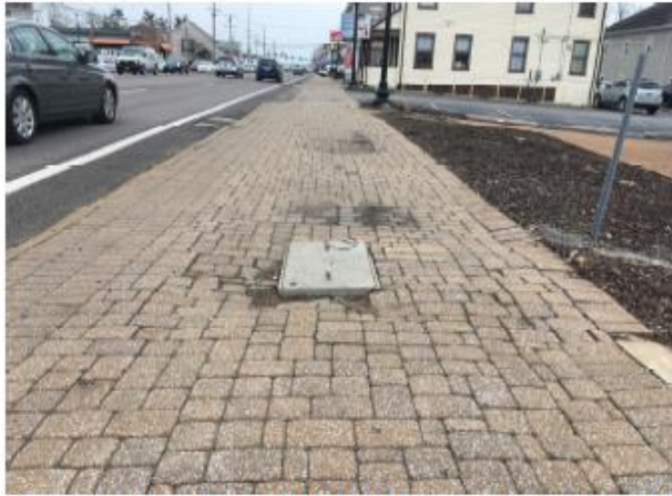
The existing sidewalk, on the South side of Manchester, does not maintain a uniform grade and has numerous vertical changes in level. These deficiencies will be corrected with a new 6' concrete sidewalk from Baxter Rd. to Hwy 141. Utility boxes will be adjusted as needed.
