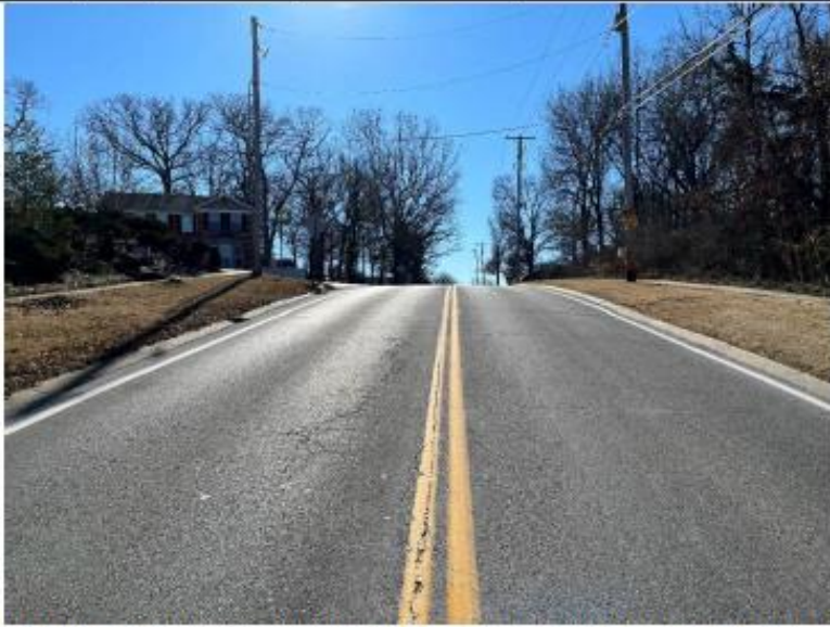
Existing Hanna Road pavement (to be milled and overlaid with an 2" Asphalt Surface)
