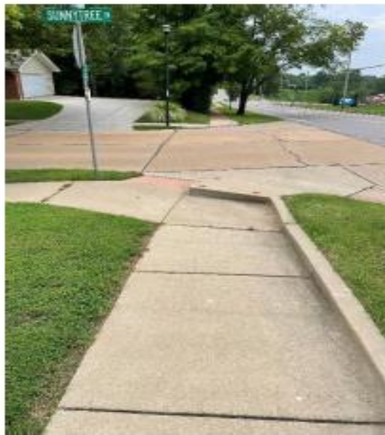
Non-ADA complaint curb ramps (on the south side of Carman) will be replaced
