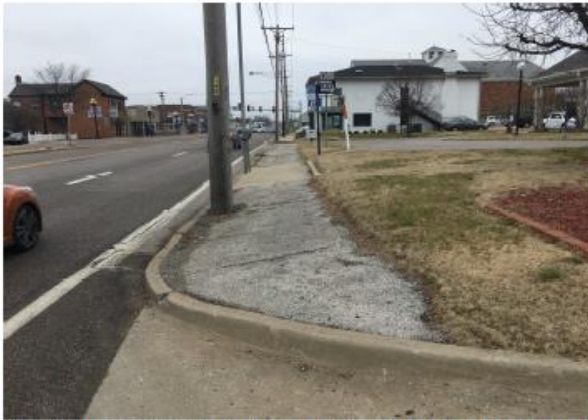
A few short, but non-contiguous sections of sidewalk/asphalt shoulder, do exist along the north side of Manchester Road. These sections are non-ADA compliant and collectively do not establish a sidewalk system.
