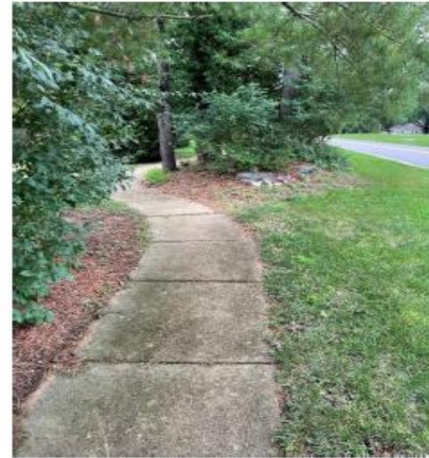
Existing 4' wide sidewalks (on the south side of Carman) will be replaced
