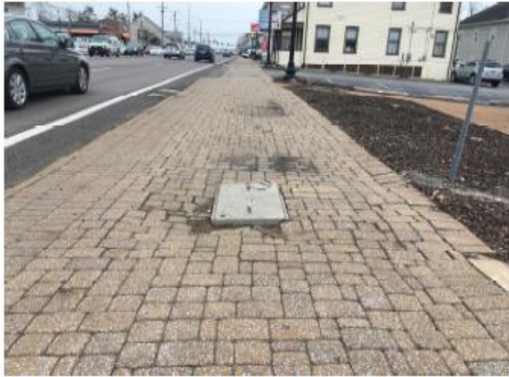
The existing sidewalk, on the South side of Manchester, does not maintain a uniform grade and has numerous vertical changes in level. These deficiencies will be corrected with a new 6' concrete sidewalk from Baxter Rd. to Hwy 141. Utility boxes will be adjusted as needed.
