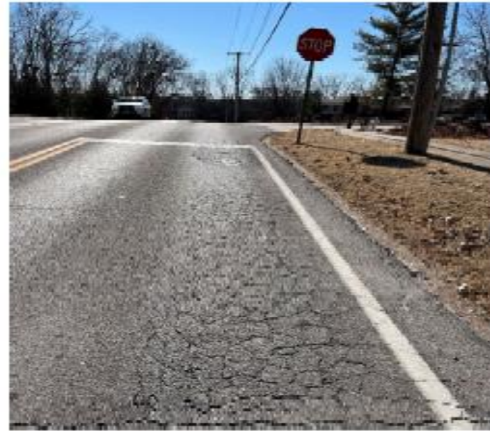
Some sections of Hanna Road will need full depth pavement repair
