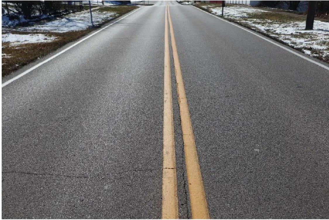
Existing Hanna Road pavement (to be overlaid with an Ultrathin Bonded Wearing Surface)
