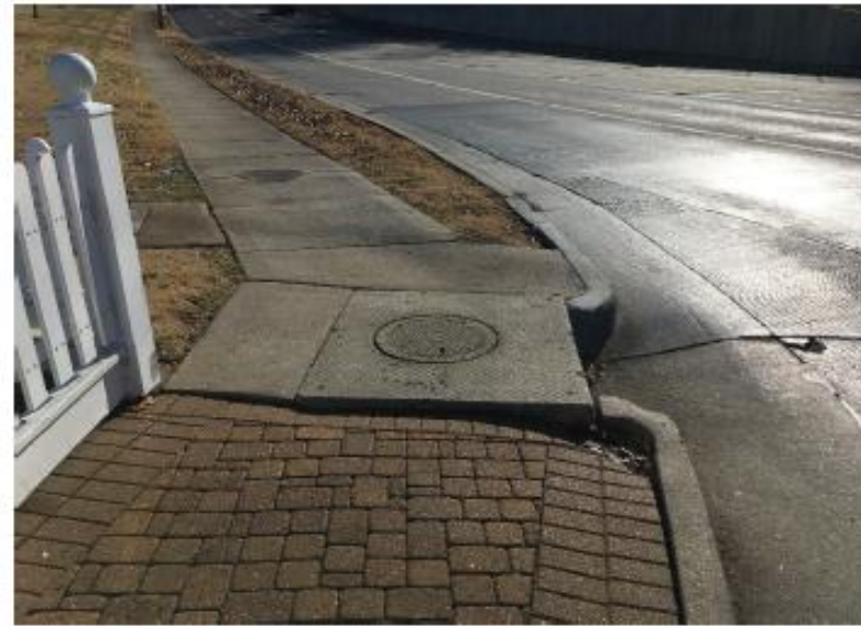
Existing sidewalk will be replaced and transitions will be made flush and free of changes in level.
