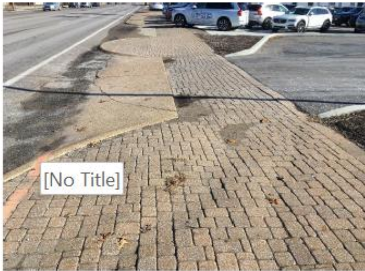
The existing sidewalk, on the South side of Manchester, does not maintain a uniform grade, nor a defined path, and has numerous vertical changes in level. These deficiencies will be corrected with a new 6' concrete sidewalk from Baxter Rd. to Hwy 141. ADA-compliant ramps and entrance approaches will be added as required.
