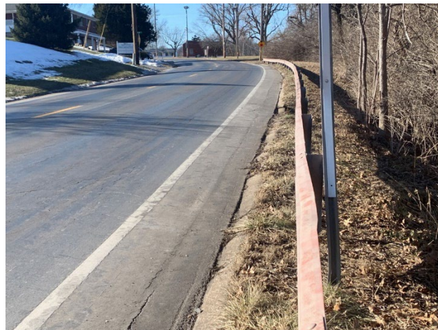
Boones Lick Road looking west towards Fairgrounds Road (no sidewalks along curve)
