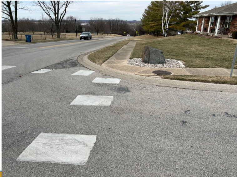
Inadequate Sidewalks and Curb Ramps
