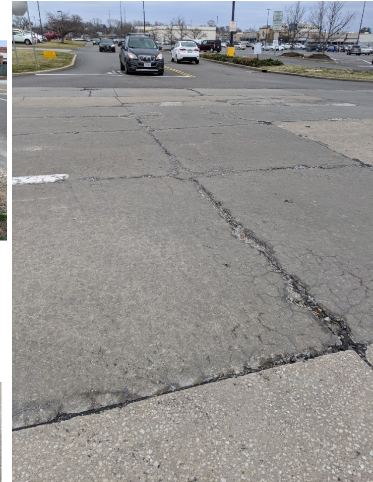
Extensive Joint Spalling
